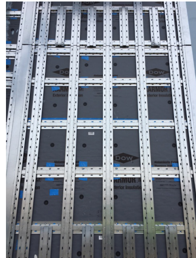
3-4. Vertical furring at 17-7/8" o.c. over horizontals. Additional vertical segments added to enable 9" o.c. Vertical Starter Track fastening. (Knight HCI™ System girts shown)
